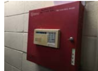
Boiler Monitoring System
