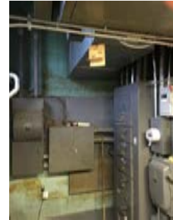
Main Electric Service
