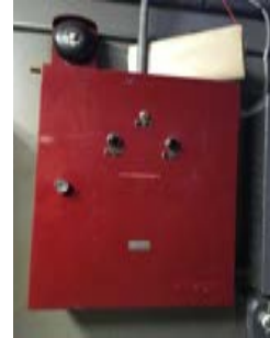
Fire Alarm Control Panel
